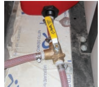
Valve position for water
